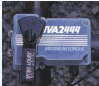
Motorised valves controls pool/ spa switching and water features
